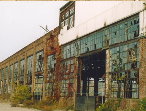
More buildings will be removed at One River Street in early summer and late fall.
